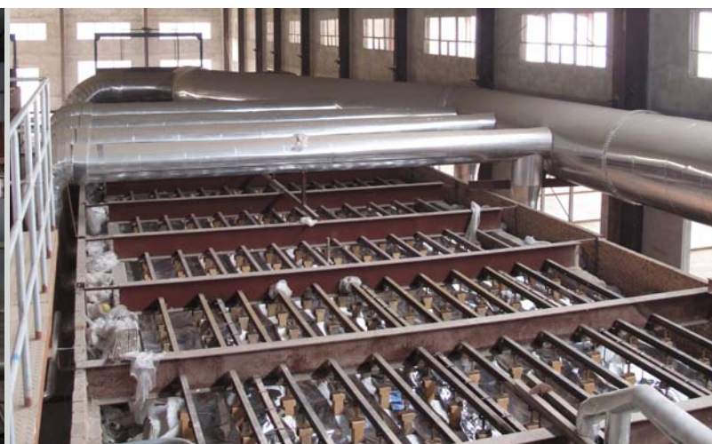
Tunnel brick kiln roof with WHRPG heat exchangers built-in at the Xinrong New Type Buildings Co. Ltd. pilot plant
