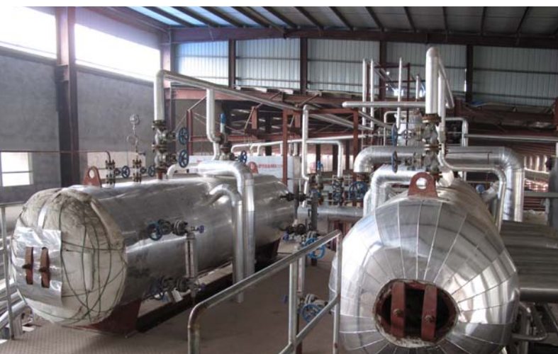
Installed WHRPG boiler components at the Xinrong New Type Buildings Co. Ltd. pilot plant
