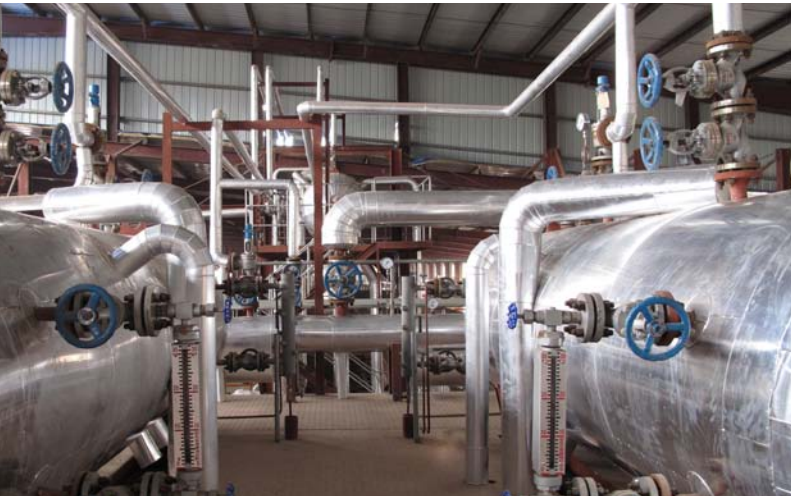
WHRPG boiler stages at the Xinrong New Type Buildings Co. Ltd pilot plant
