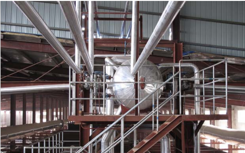
Main WHRPG boiler at the Xinrong New Type Buildings Co. Ltd. pilot plant
