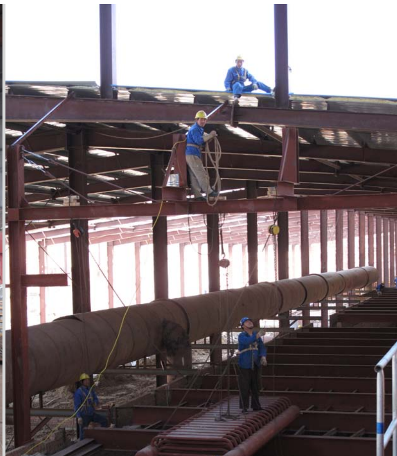
Installation of WHRPG components at the Xinrong New Type Buildings Co. Ltd. pilot plant
